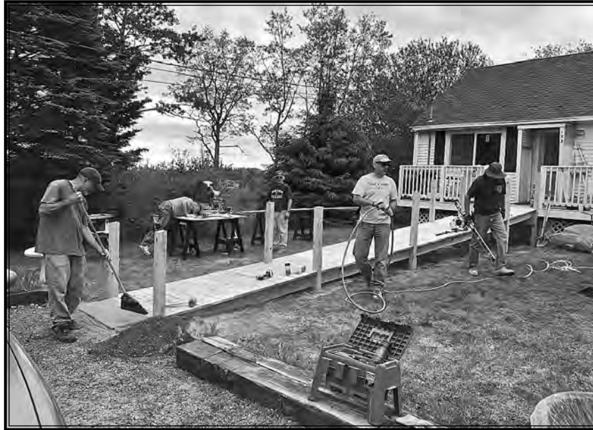
The Maine Seacoast Mission's Housing Improvement program helps Downeast homeowners keep their homes accessible, warm and dry. MSM photo.
